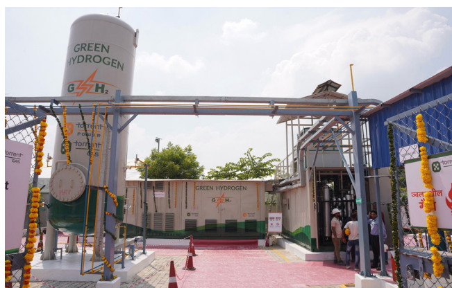
Torrent Power's state-of-the-art Green Hydrogen Production Facility at Gorakhpur
